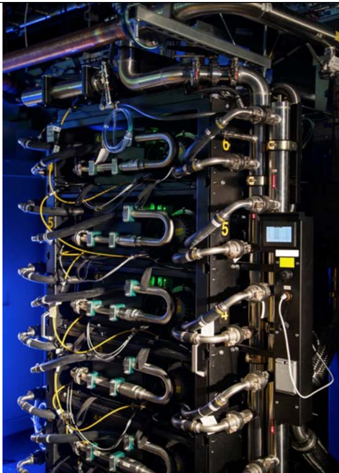
Figure 14: TPU v8 has upgraded to fourth-generation (Gen4) liquid cooling CDU
