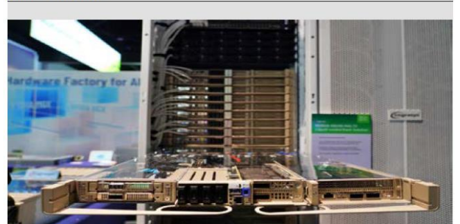
Figure 6: Side view of Hon Hai's GB200 NVL72 liquid-cooled rack solution
